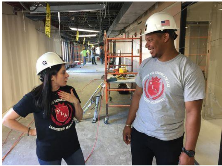
Principal Nicole Fama and Director of Operations Javaris Carrion talk on June 19 inside the new Phalen Leadership Academies Middle School. The school, now undergoing a renovation, will open to 7th- and 8th-graders in July. (Photo: Matthew Tully)
